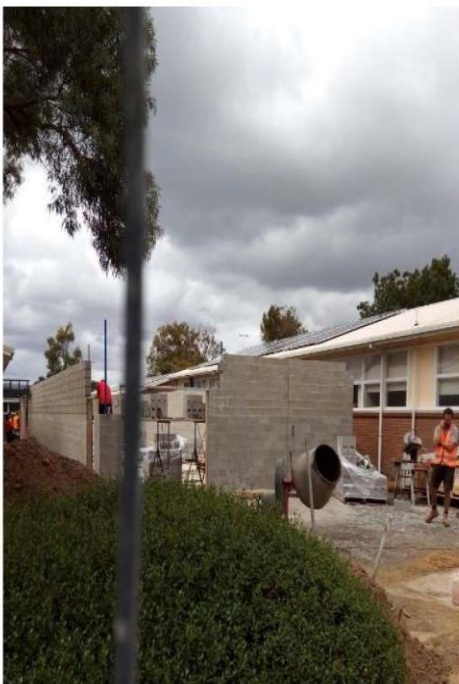
Front view. Shed entry will be to the left of the building; the large gap in the front will be filled by a roller door.
